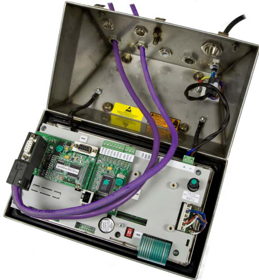
Figure 2-42: PROFIBUS Cable Connection in Harsh Enclosure
