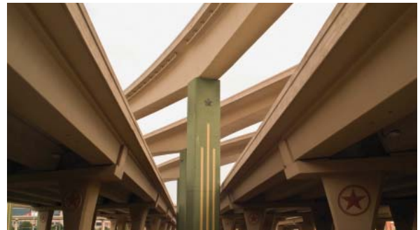
Orthotropic ribs are used in the High Five interchange in Dallas, Texas.
