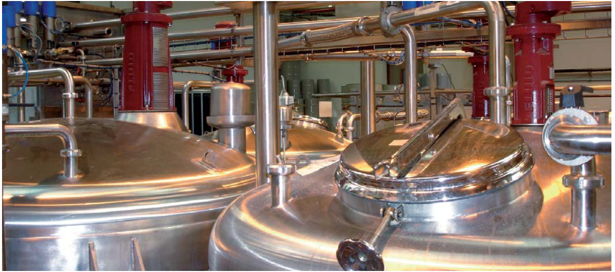
Tanks with multiple attached pipes
