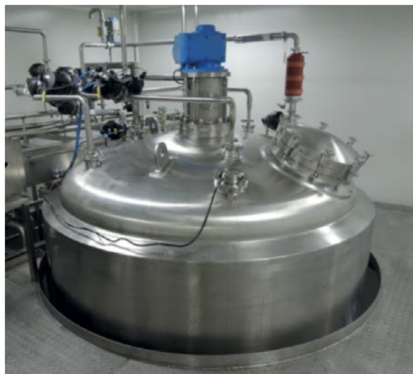
The reactor's upper section extending through the next floor with adequate space for movement
