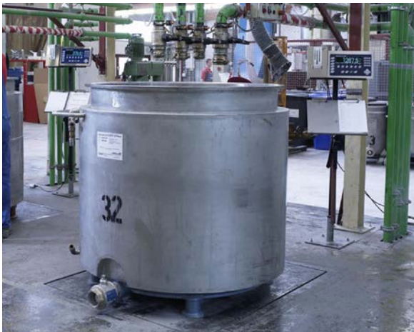
Tank with pipes unattached
