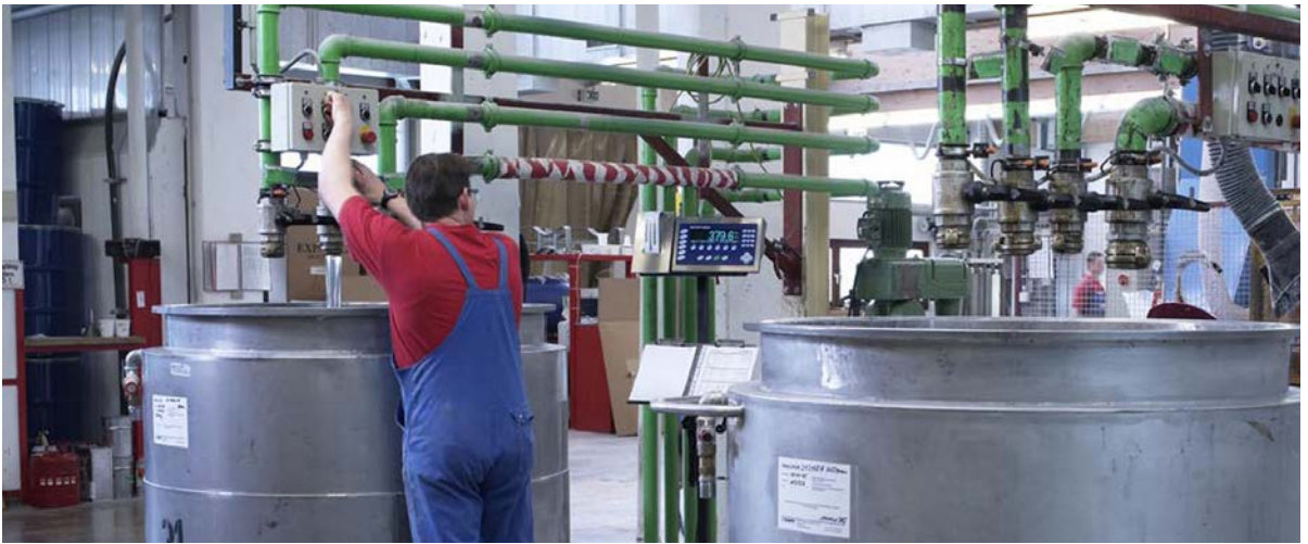
Figure 27: Manual Filling Operation
