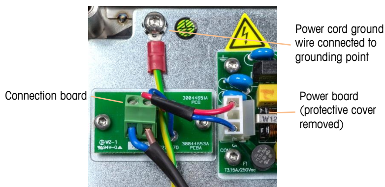
Figure 2-18: IND236 AC Power Connection Board and Grounding
