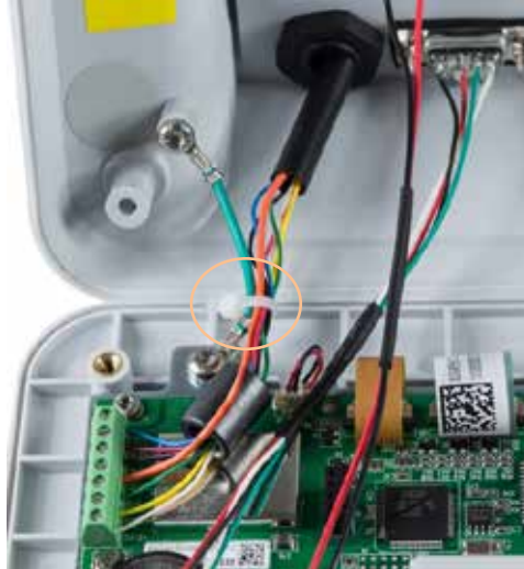
Figure 2-20: Analog Load Cell Pin Grounding and Ferrite Installation, IND231
