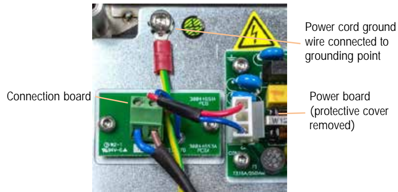
Figure 2-18: IND236 AC Power Connection Board and Grounding
