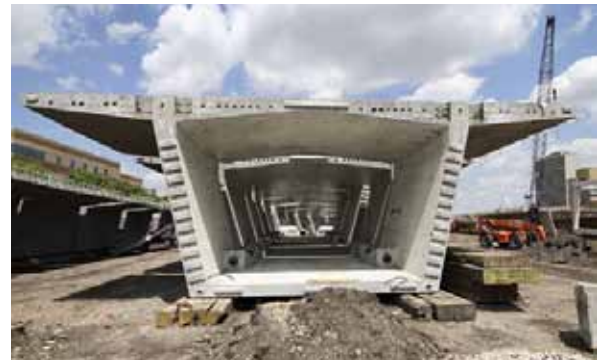
Minneapolis I-35W Bridge replacement uses a closed orthotropic rib to support the deck. This design was chosen after the previous I-beam bridge collapsed in 2007. (Photo courtesy of http://www.nytimes.com/imagepages/2008/06/08/us/08bridgex.ready.html )
