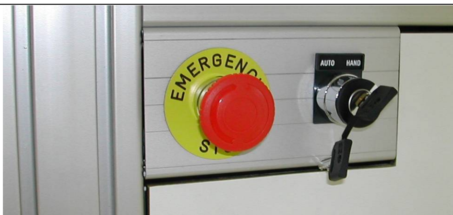
Figure 3 Panel with „EMERGENCY“ push-button and „AUTO / HAND“ key-switch
